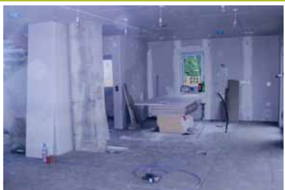
Hanse fitted the wiring and plumbing so that Tony could concentrate on the finishing touches
