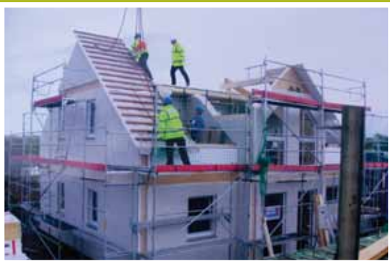
Once the roof was in place, the house became watertight and ready for internal works
