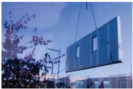
The wall panels were craned into position and the house quickly begins to take shape
