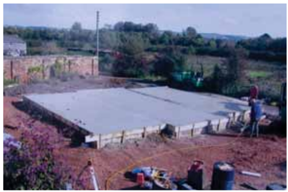
Groundworks begin on site, and the foundations were put in place by September 2008, ready for the build
